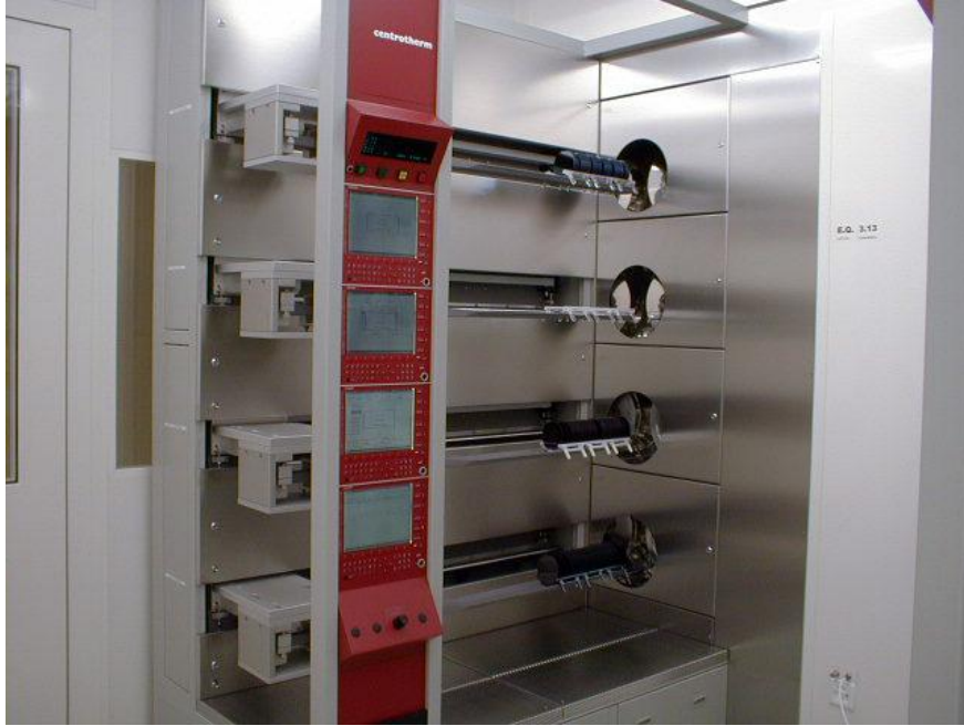
Centrotherm furnaces, 15 tubes in 4 stacks
